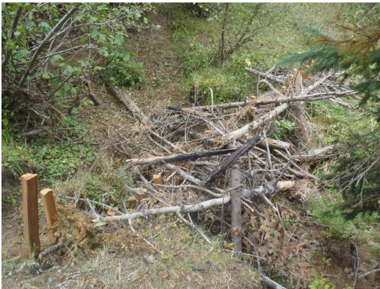
Figure 1. Corral Creek FBD After Installation
